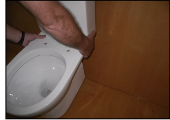
3 – With reference to the sewer hole, center the basin where it will be.
